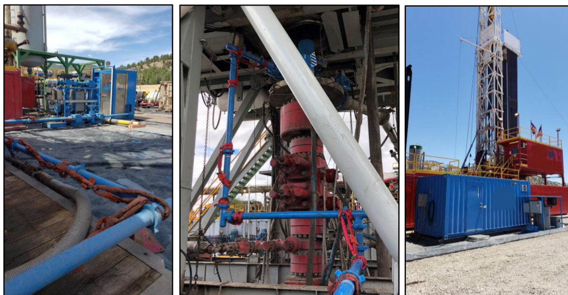
Figure 12—MPD choke system and Coriolis meter (left), RCD and MPD flowline (center), and MPD control center and tool shack (right)
