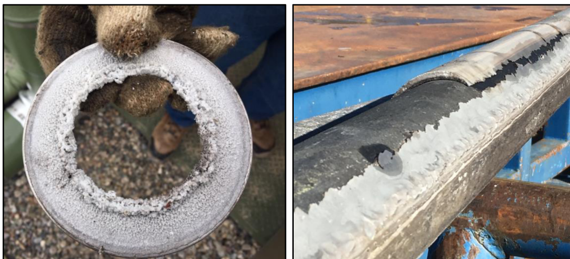
Figure 15—Left scale build-up in top side facilities, right scale build on completion
